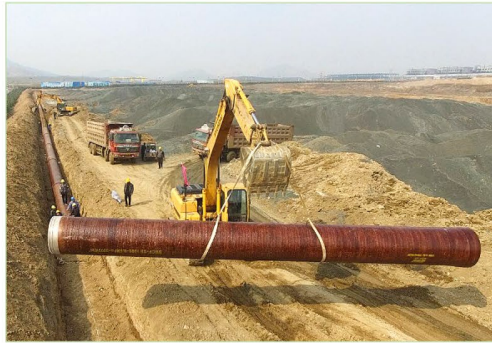
Drinking water pipe
